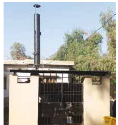
NEW INSTALLATION - MEDICAL WASTE INCINERATOR
